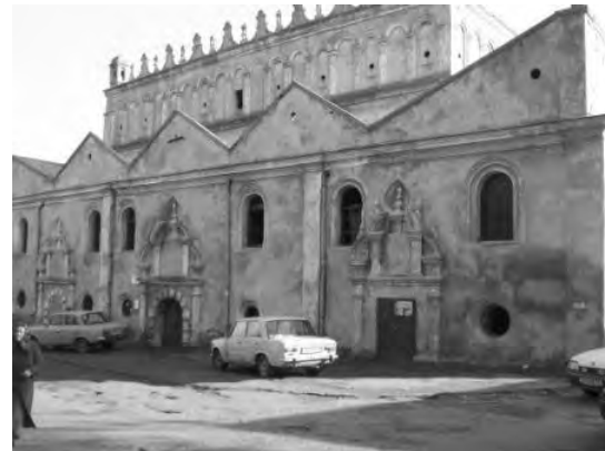
Synagogue in Zhovka, Ukraine, which is currently abandoned and occupied by the homeless despite designation as a protected site
