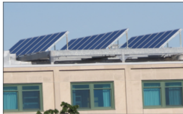
20 KW SOLAR PHOTOVOLTAIC ROOFTOP SYSTEM
