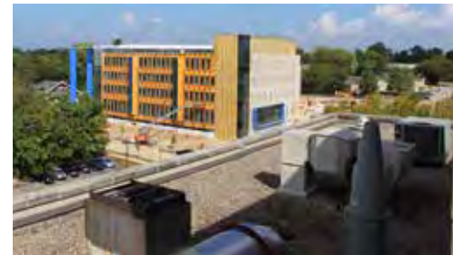
View of Luddy Hall under construction, looking west from the roof of the Geology building.
